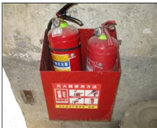
Photo of fire safety equipment Fire extinguishers.JPG
