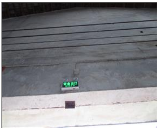
Photo of fire safety equipment Exit sign.JPG
