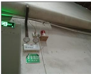
Photo of fire safety equipment Fire alarm with backup power.jpg
