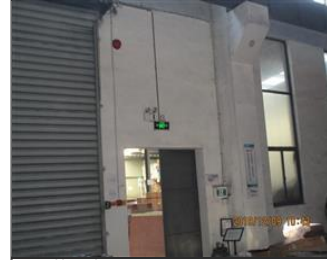
Photo of fire safety equipment Emergency lighting and exit sign and fire alarm.JPG
