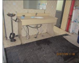
Photo first aid facilities Eye washer.JPG
