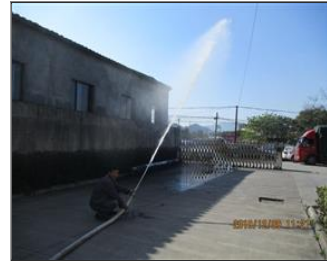
Photo of fire safety equipment Hydrant testing.JPG
