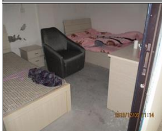
Photo of non-conformity The room at the roof for person living.JPG
