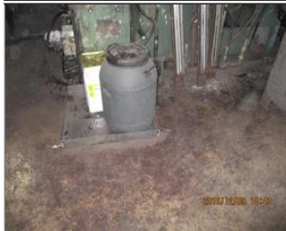
Photo of non-conformity No safety label.JPG
