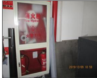
Photo of fire safety equipment Hydrant and fire extinguishers.JPG
